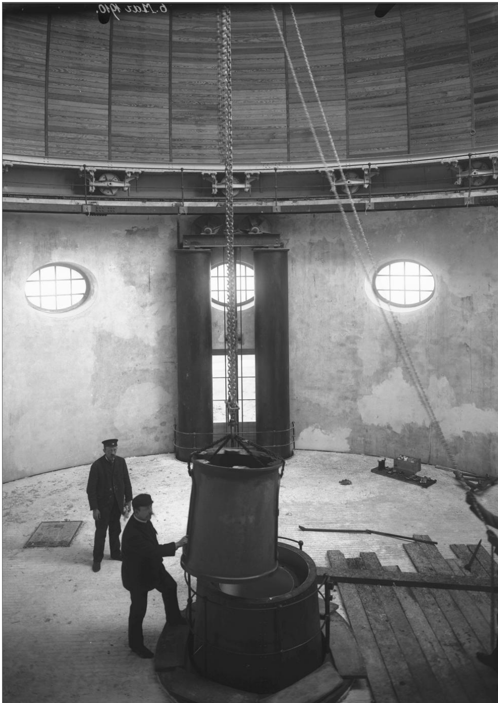
Figure 3: Construction work on the mount for the Great Refractor telescope in March 1910. Credit: Photographic Archive of the Hamburg Observatory
