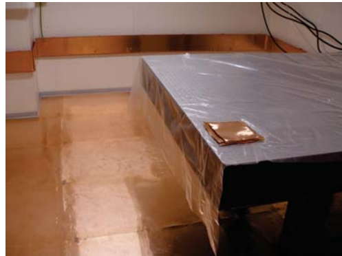
(b) Interior view during construction 1. The central ground plane for the room is a copper band attached to the wall.
